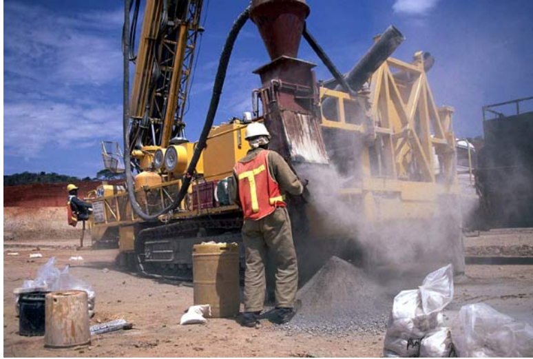
Figure 3: Exploration drilling operations. Note the masking system, helmet, field boots, which are essential components for personal safety
