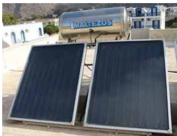
Solar thermal system for water heating
