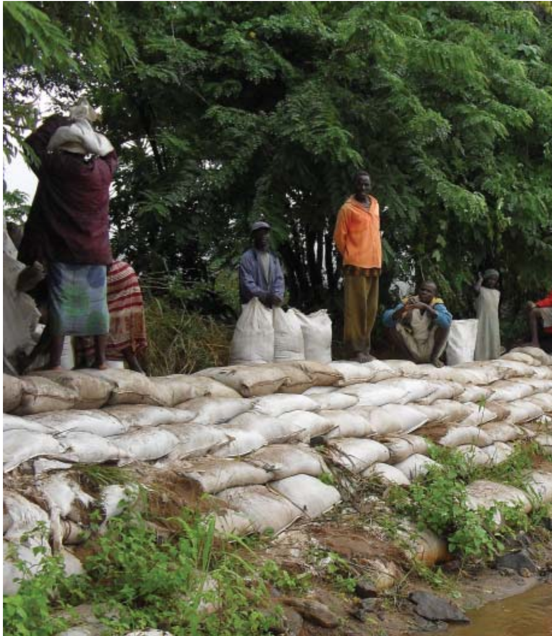
Construction of dykes on the Lalanje river in Nsanje District. The initiatives are in line with Component II, Disaster Risk Management, Climate Change and Environmental Sustainability
